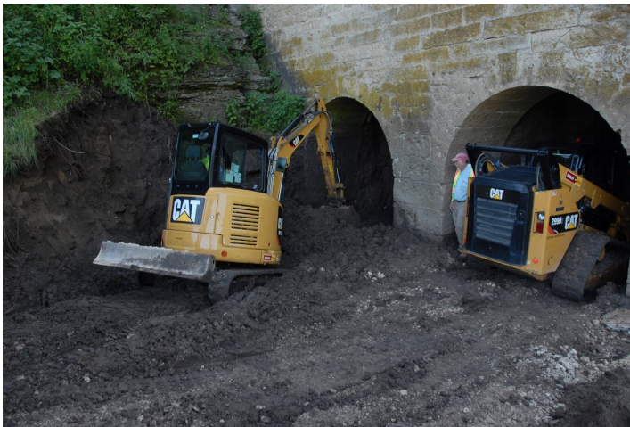
Chris Schoen watches C. J. Moyna employees enter the basement arches to begin removing sediment from the Motor Mill Basement.
