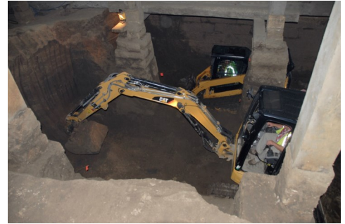
C. J. Moyna employees use a mini-excavator and skid loader inside the Motor Mill basement to remove sediment.
