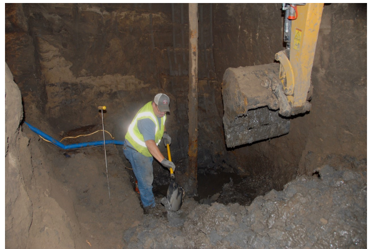
C. J. Moyna employee Bryan Willson digging in the mud to allow the removal of a turbine from the basement.
