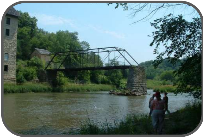
Half of bridge was destroyed during the flood of 1991, the other half was destroyed during the flood of 2008
