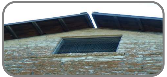
Gap in peak before 2009 joist and roof replacement
