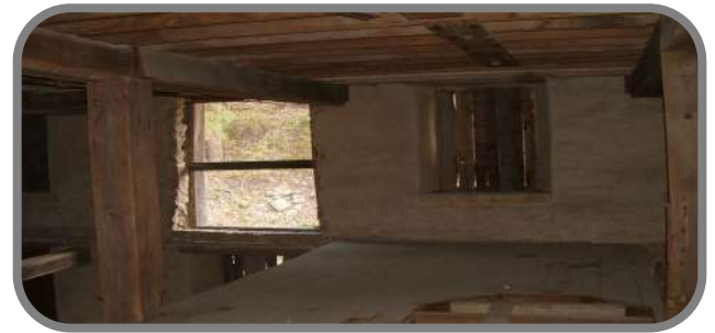
Previous to major window replacement
