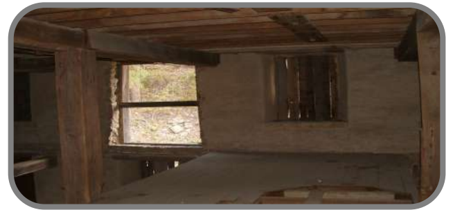
Previous to major window replacement
